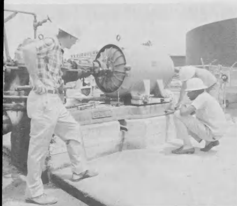
Aligning a motor-driven centrifugal pump, using clamp-on jigs which allow rapid "hot" measurements without requiring coupling separation. Alineamiento di pomp centrifugal y motor, usando "clamp-on jigs" cu ta permiti midimento di "calor" rapido sin desconecta e mashinnan.
